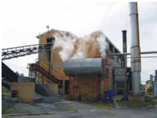
CONDENSATE RECEIVER TANK BEFORE
